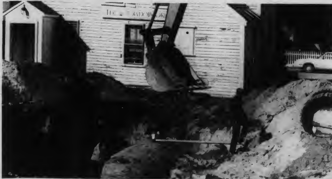
A giant hole was dug behind the Bowdoin Orient, in the Physical Plant parking lot, to replace an 18-year old, 10,000 gallon fuel tank with a new 6,000 lbb. fiberglass tank. Photo by Asaf Farashuddin.
